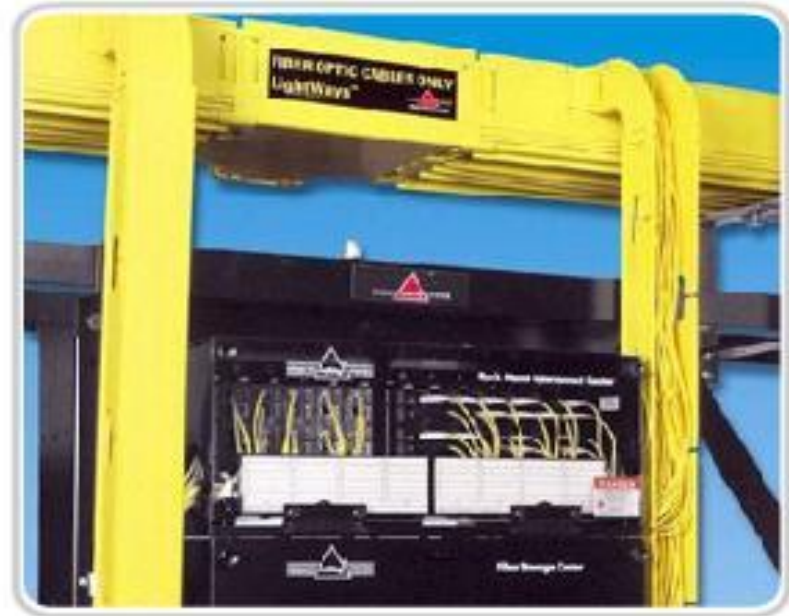
Fiber Cable Raceway
